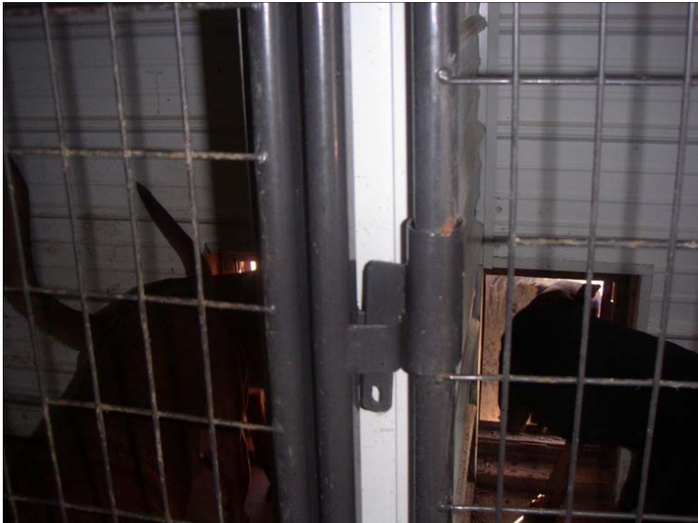
Rusty Metal and Broken Dog Door
