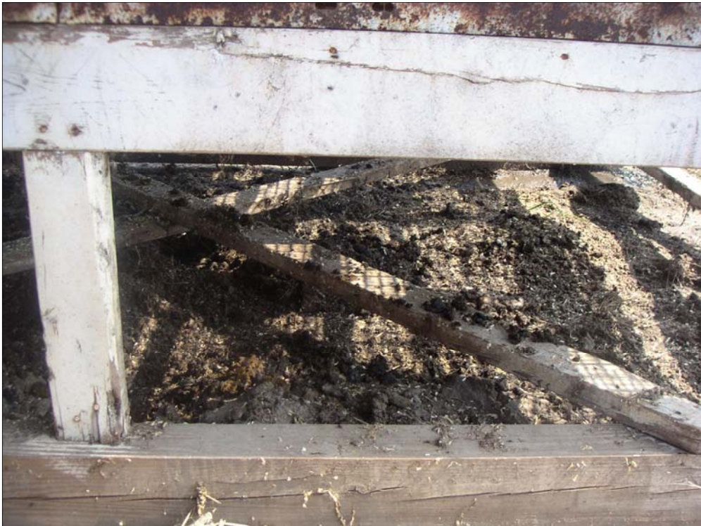
Fecal Accumulation and Worn, Cracked Wood
