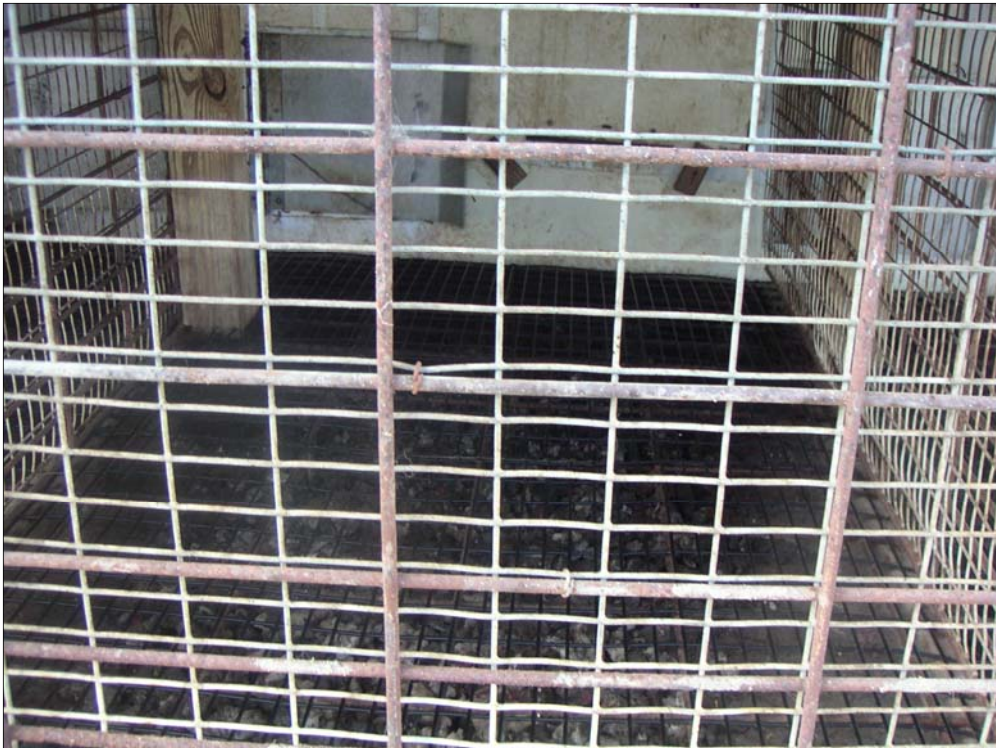
Fecal Accumulation, Rusty Metal and Dirty Walls
